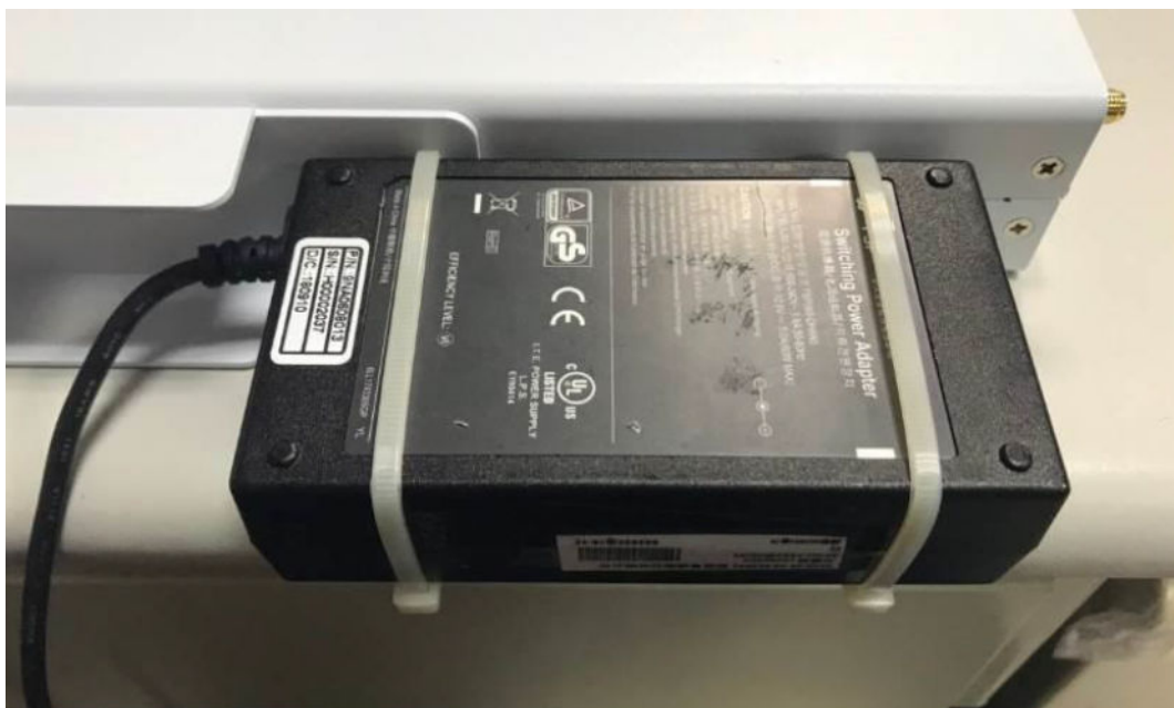
Figure 15: Secure External Power Supply
