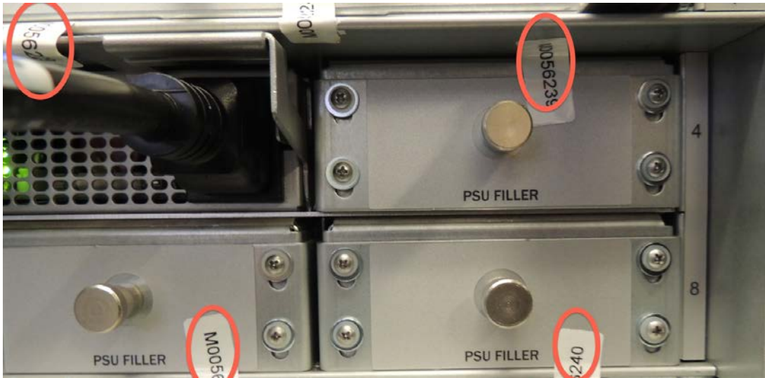
Figure 5. Seal locations on the port-side of the VDX 8770-8
